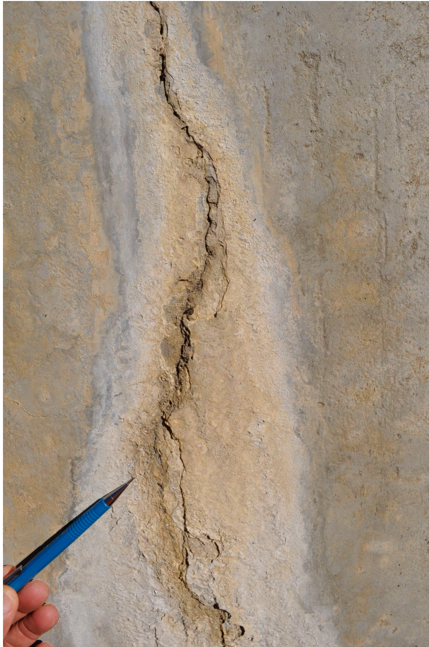
Photograph 13. A close-up of a typical leaky crack with rust-like brownish stains.
