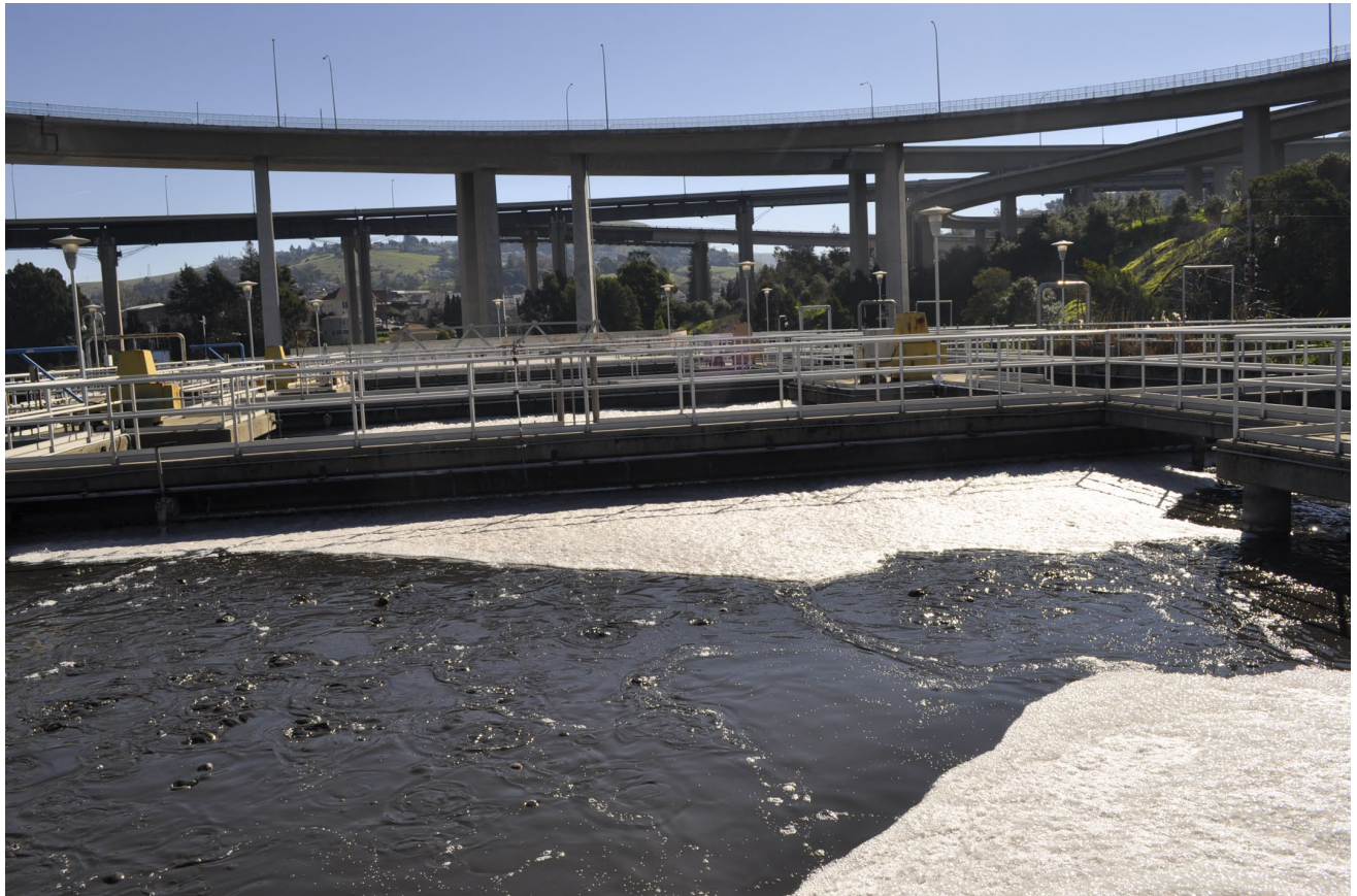
Photograph 15. An overview from the top of the structure. The visible portion of the concrete elements did not show substantial distress.
