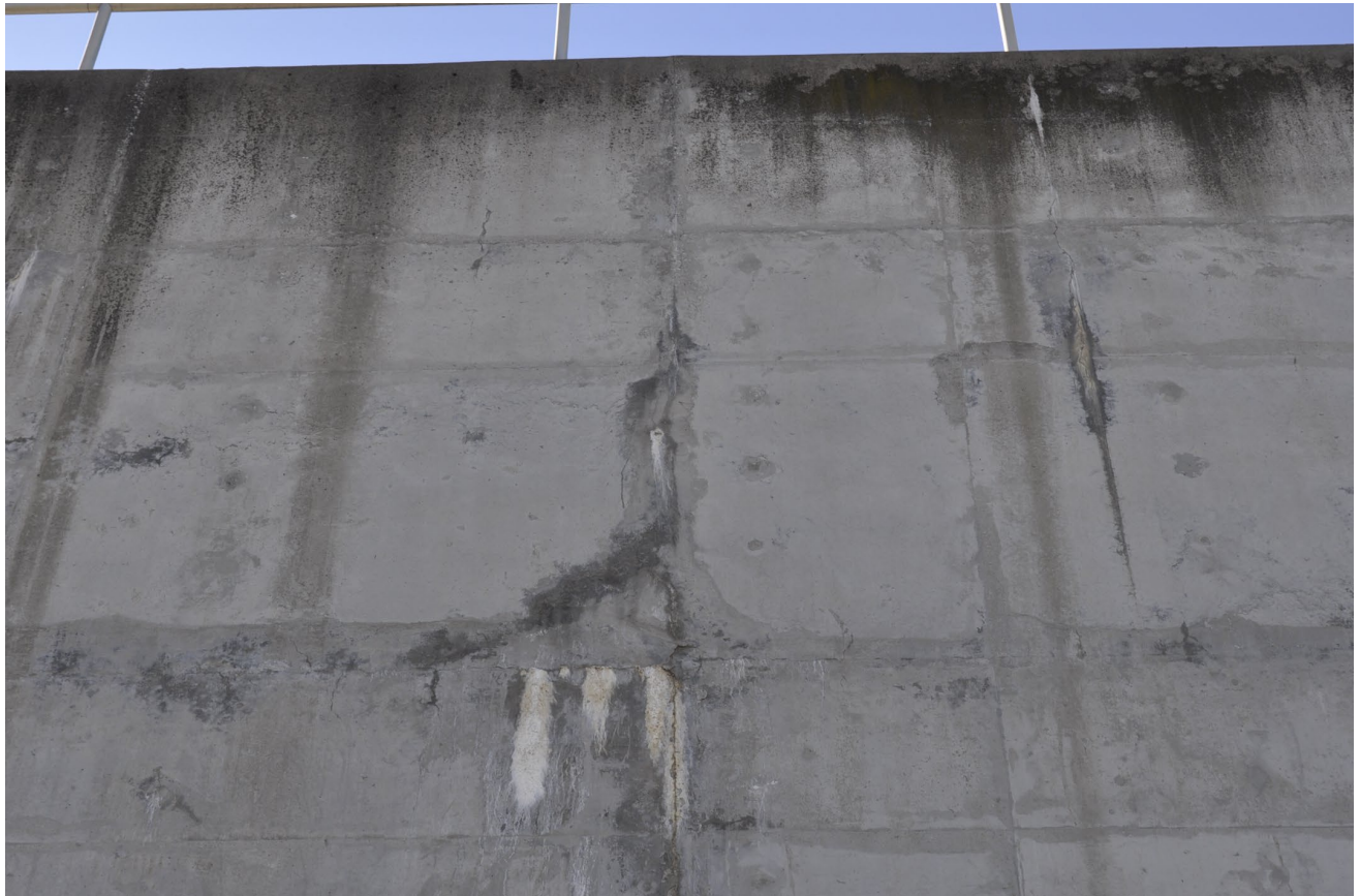
Photograph 12. Another location shows a sewage water leak through vertical and horizontal cracks and efflorescence.
