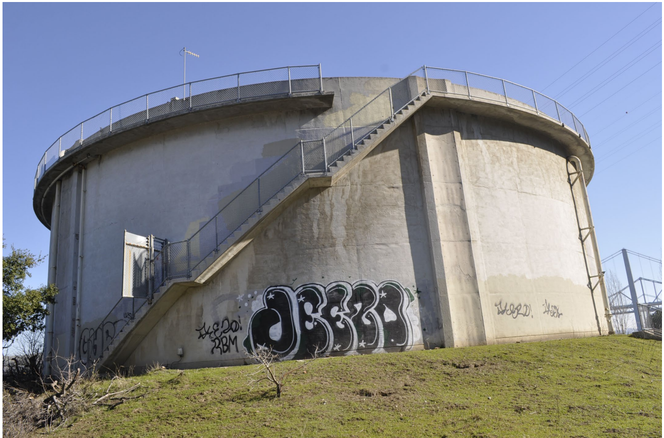
Photograph 1. An elevational view of the circular sewage tank with a staircase to reach the top of the tank.
