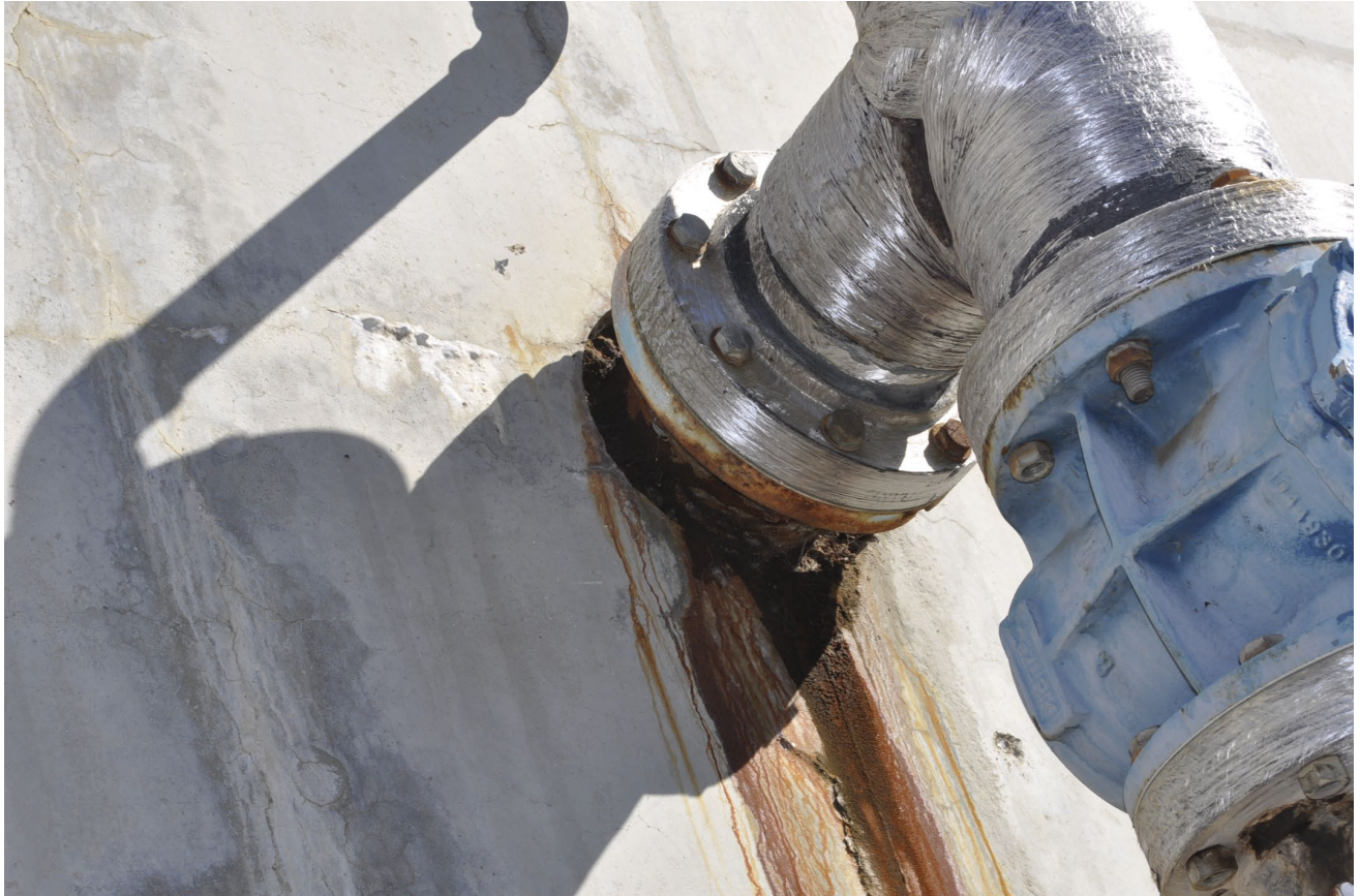
Photograph 14. Rusty pipe. The leak staining the wall with rust stains.
