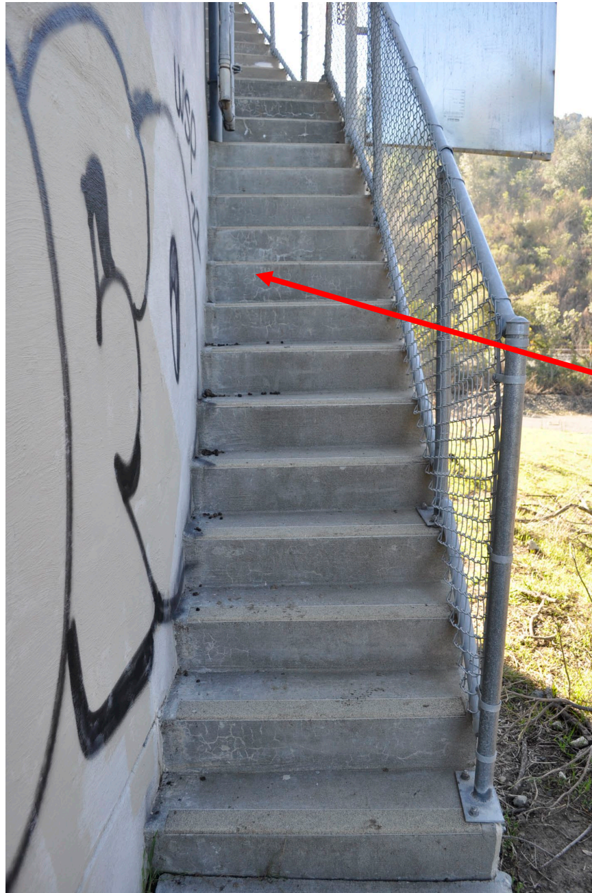
Photograph 3. The lower section of the staircase shows cracking and efflorescence.
