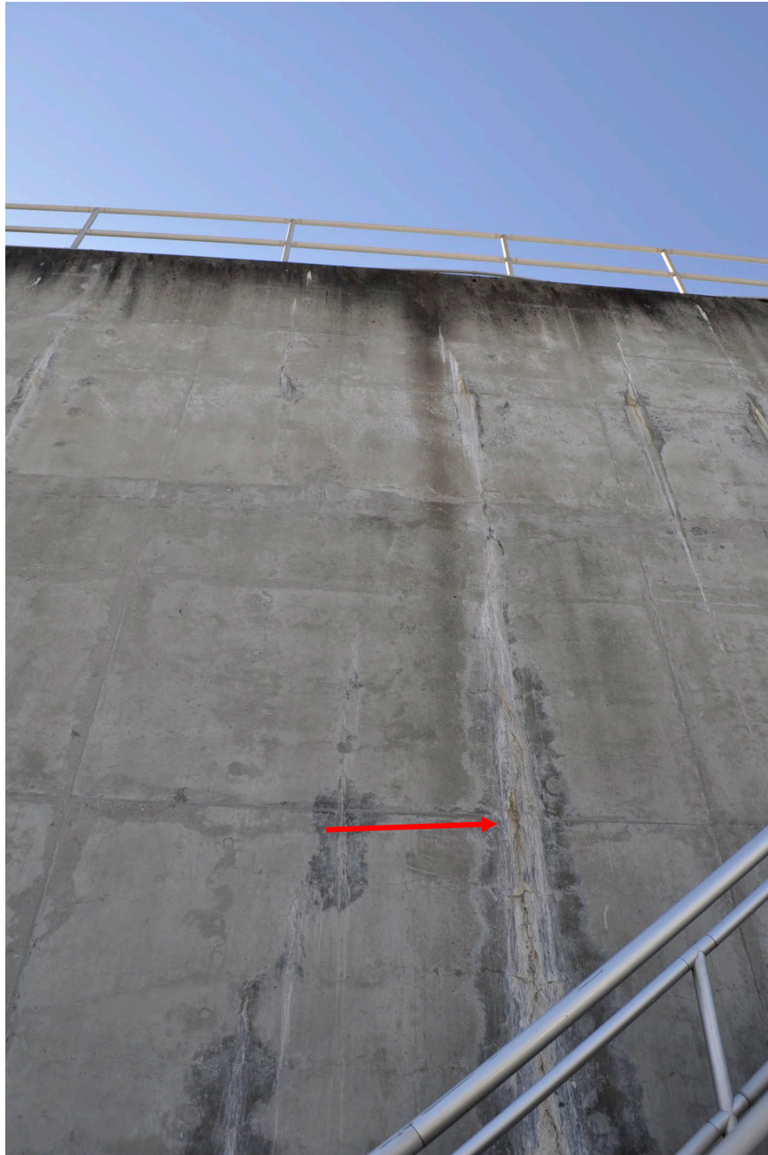
Photograph 11. Another long wall of the structure showed a sewage water leak and reinforcement rust-like stains along the leak.
