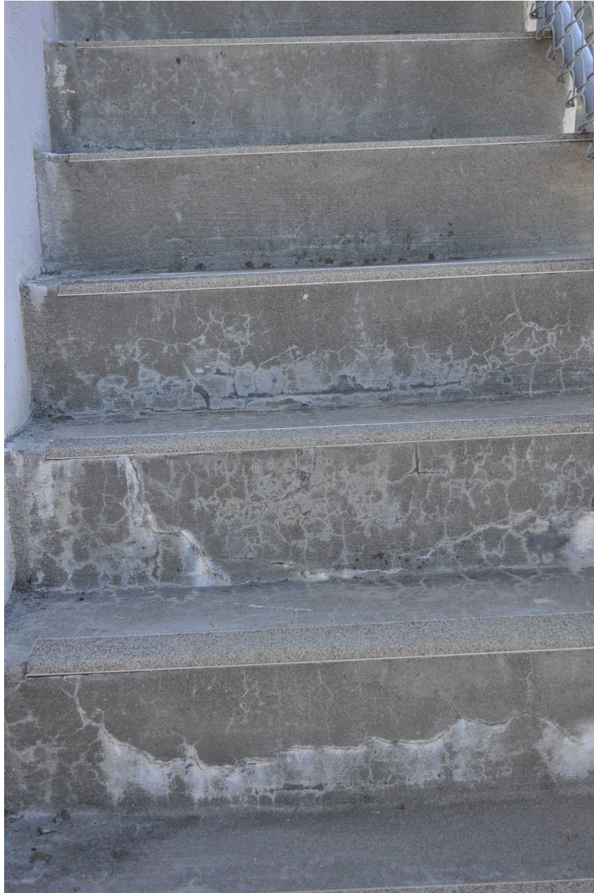
Photograph 4. Close-up of cracks in stairs with white efflorescence.
