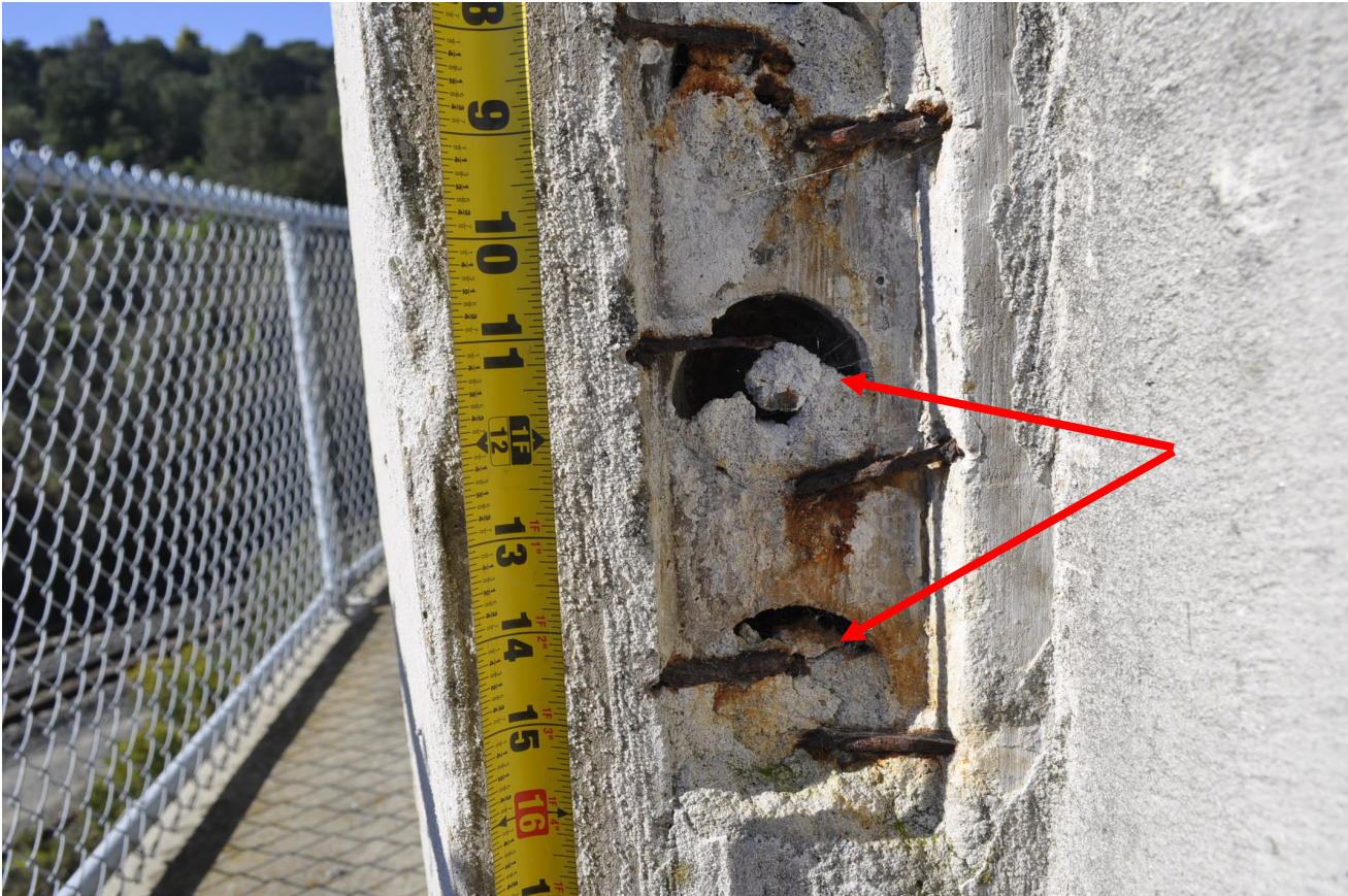
Photograph 8. The close-up of corroded nails and post-tension anchor pockets (red arrow).
