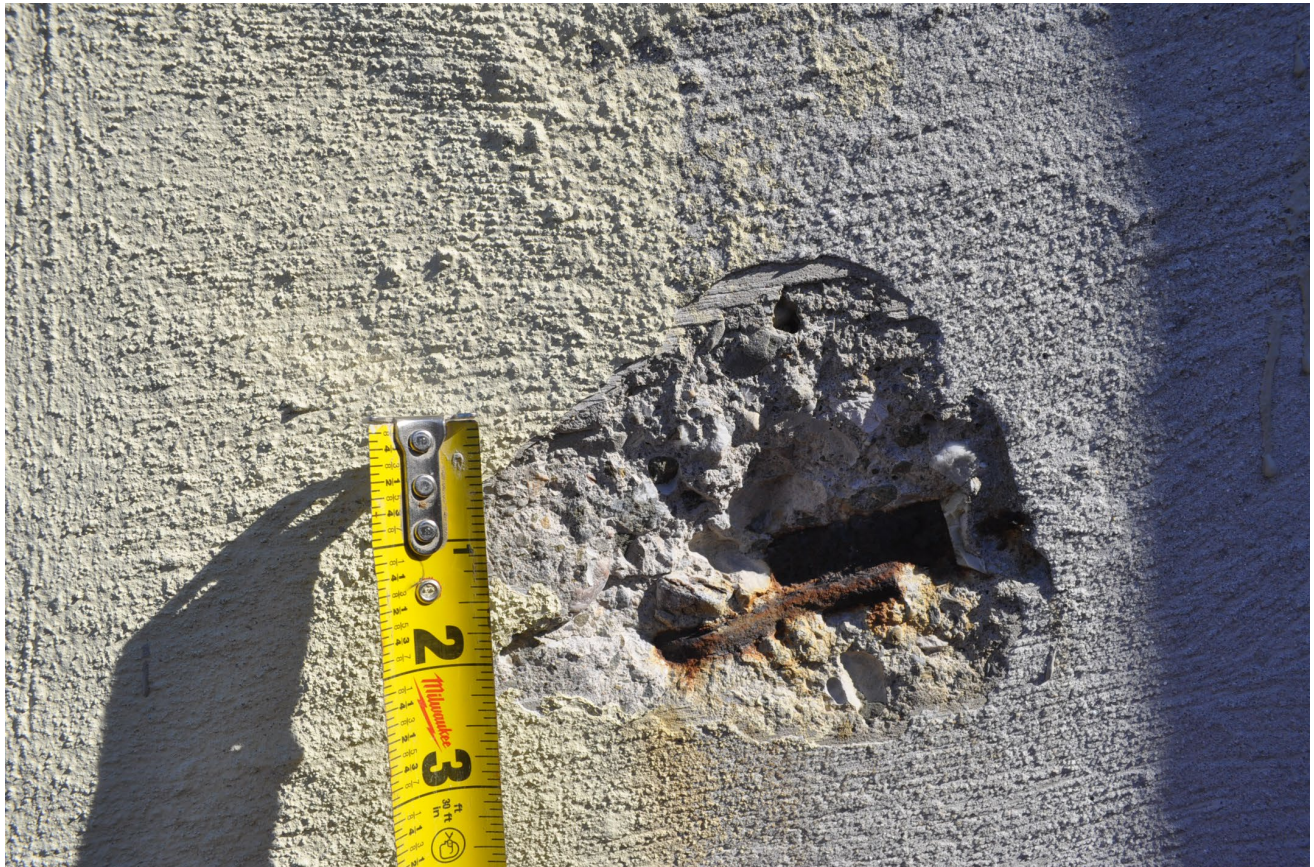
Photograph 5. Close-up of corroded reinforcement in the wall.
