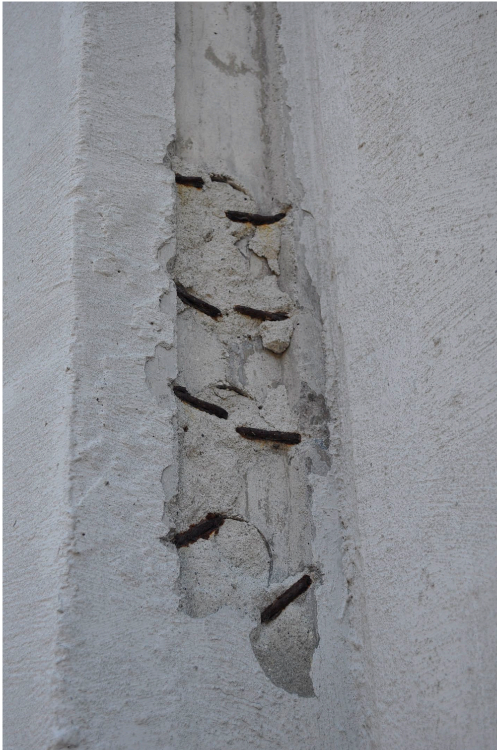
Photograph 2. Corroded nails or part of reinforcement was corroding in the pilasters.
