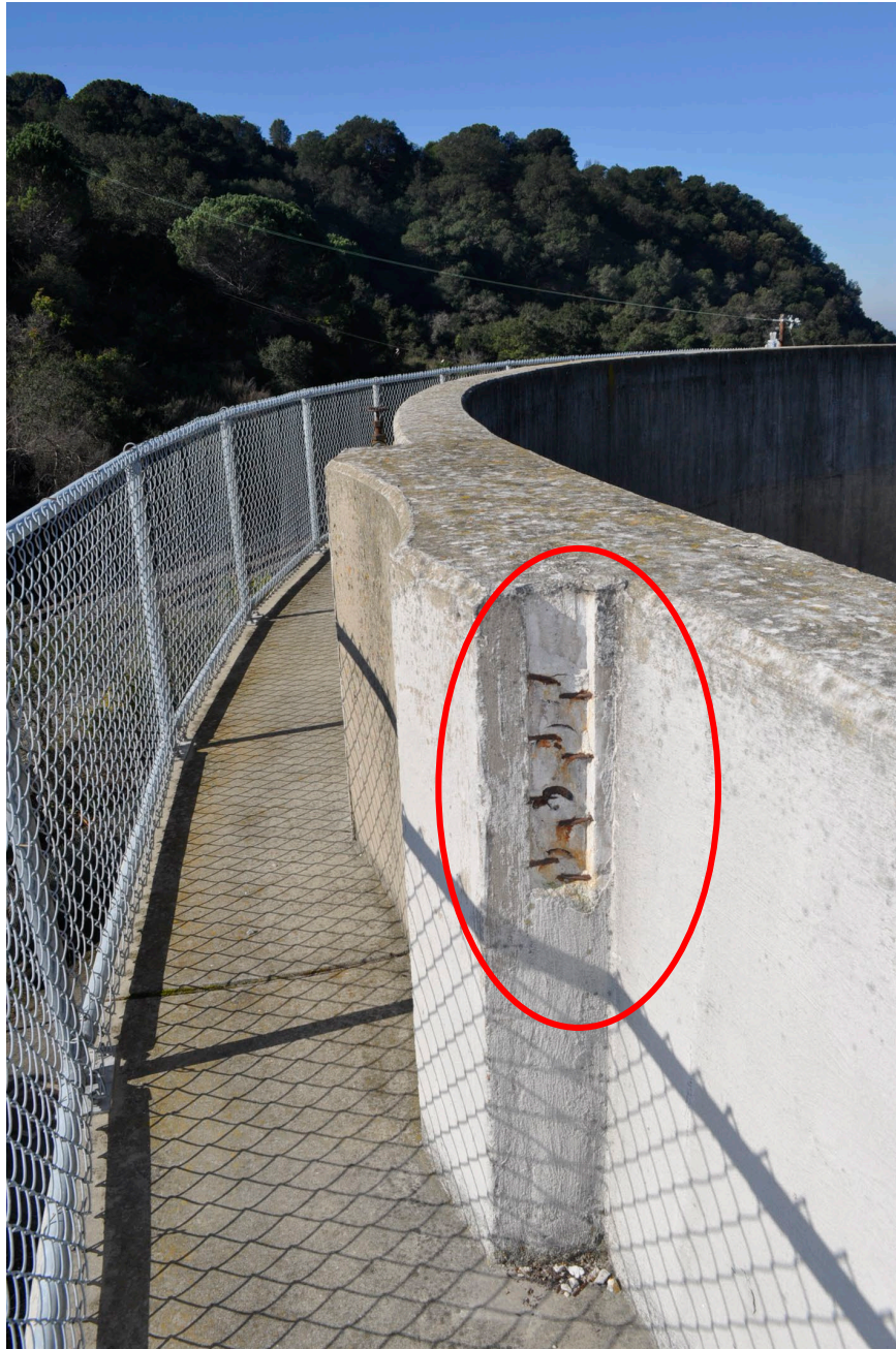
Photograph 7. The pilasters showed corrosion of metal.
