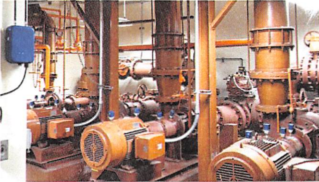
Sensors placed on specific points of the pump based on application. The sensors are connected through low-energy Bluetooth to a node placed on the wall. The node utilizes a cellular gateway to transmit data to cloud.
